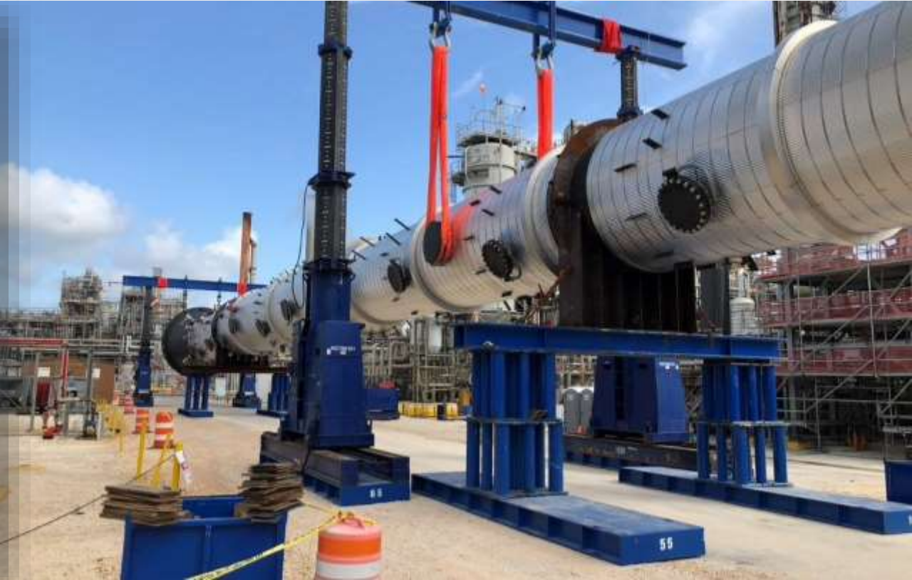
378,000lbs Recovery Column
